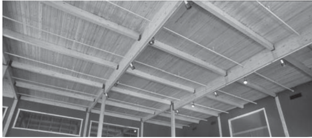
Figure 1.3 Interior of a building with a panelized roof system. (Photo courtesy of Southern Pine Council)
