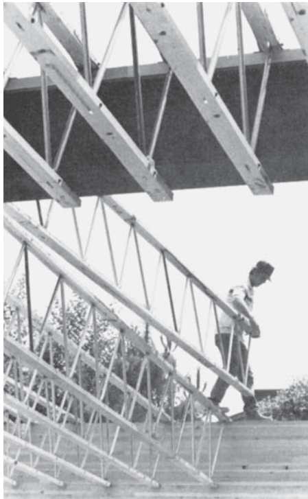
Figure 6.33a Wood trusses with tubular steel webs. Trusses in the foreground are supported on a wood member attached to a steel W-shape beam. In the background, trusses rest on glulam. (Photo courtesy of Trus Joist—A Weyerhaeuser Company).
